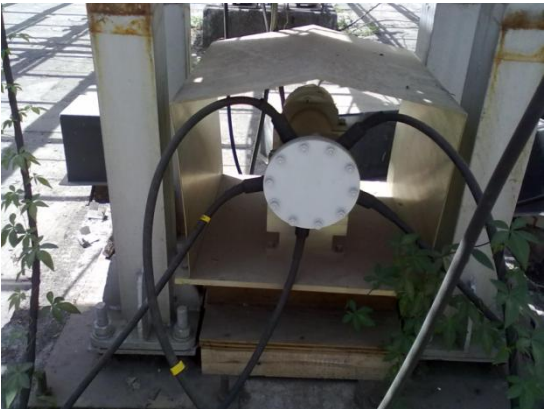
Figure 4. 1:5 way power divider/combiner placed in the field, five outputs can be seen clearly
